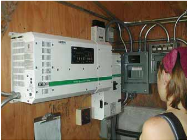
The balance of system components for a DC hydro system are very much like a photovoltaic system, except the charge controller shunts to a diversion load.
