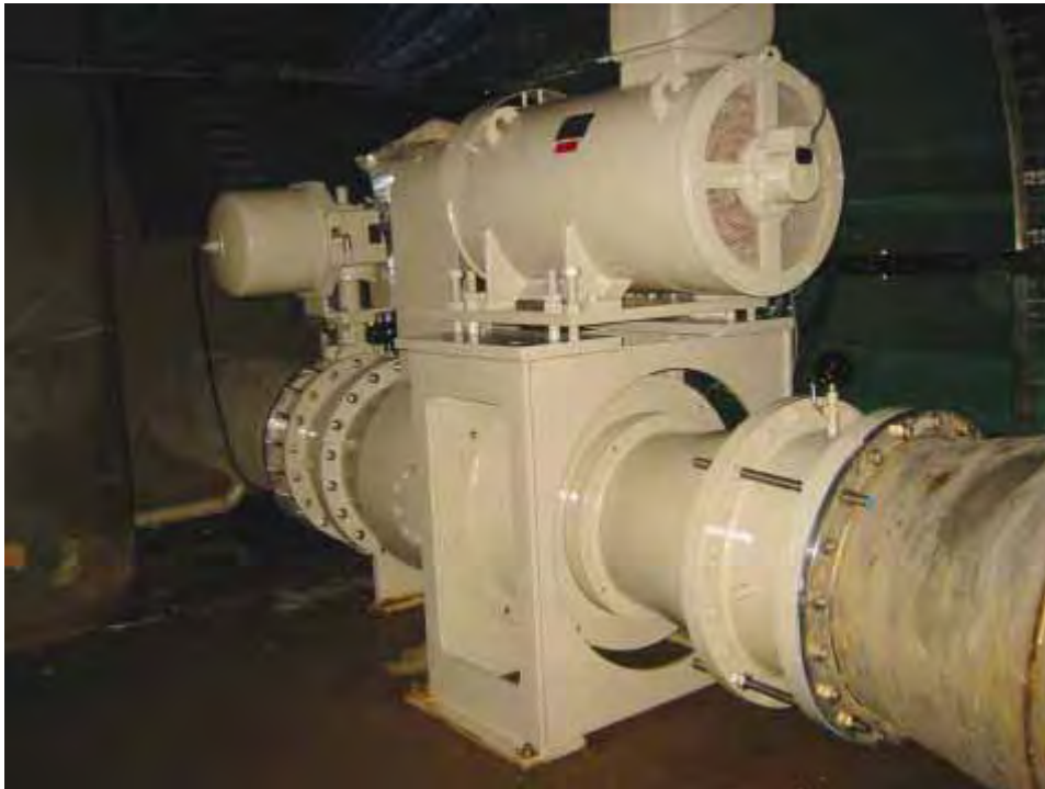
Figure 9: Taichung, Taiwan 68 kW Micro-Hydro Turbine
