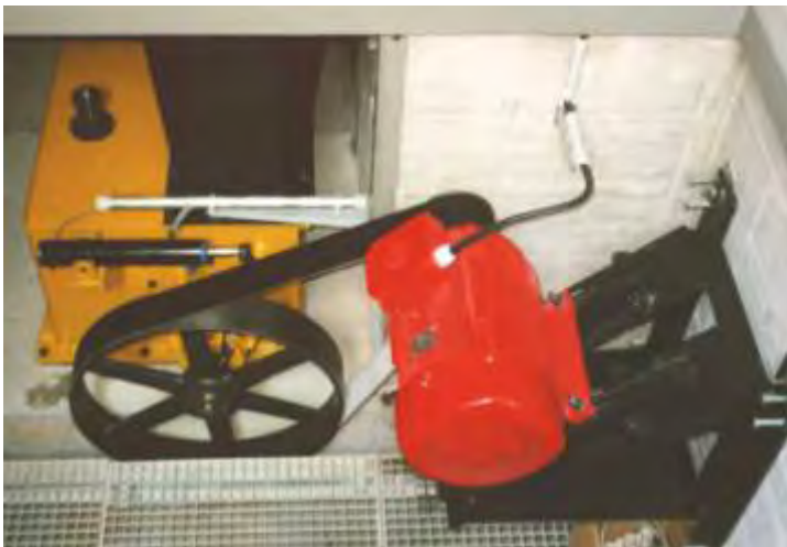
Figure 8: Emmerich, Germany Micro-Hydro Turbine
