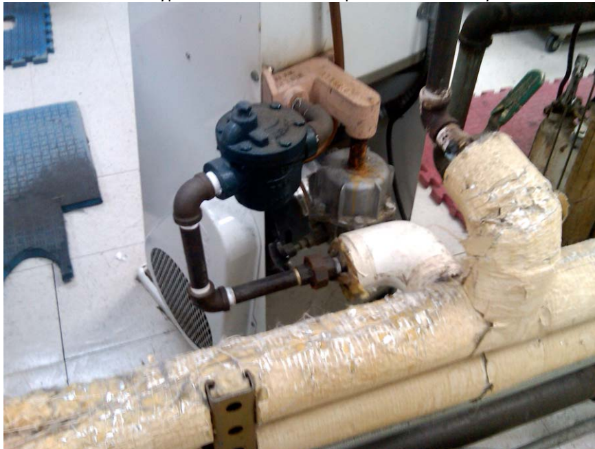
Photo 2 – Typical installed steam trap on an insulated system
