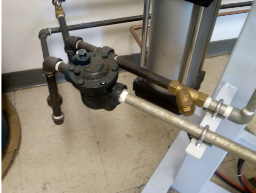
Photo 1 – Typical installed steam trap on uninsulated system
