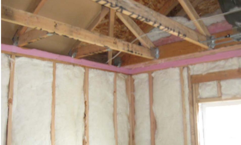
Figure 1. Photograph of sill sealer (pink band at top of wall) installed on the top plate prior to drywall installation (courtesy of Fluid Market Strategies; Manclark, 2013).
